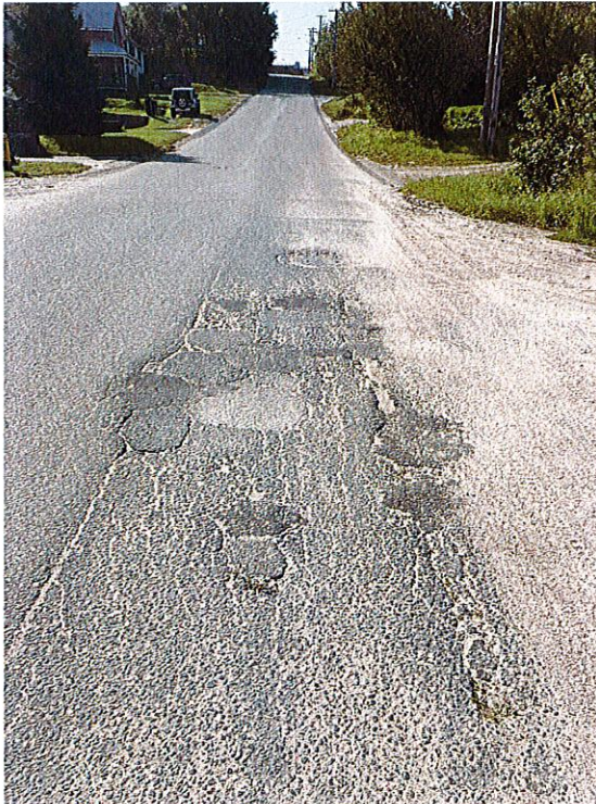
Photo 3: Example of PCI between 46 and 65
